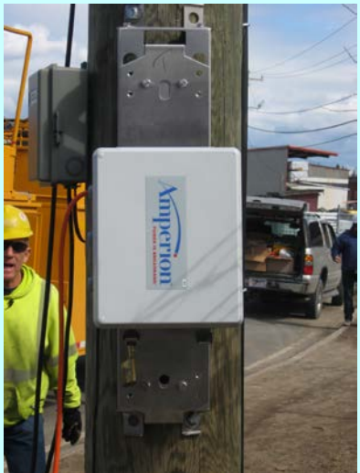
Pole Mounted PLC Modem
