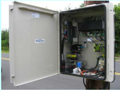
DG Recloser Unit
